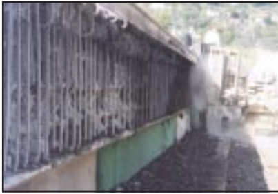
At 150 mm depth, the rebars are totally exposed.
