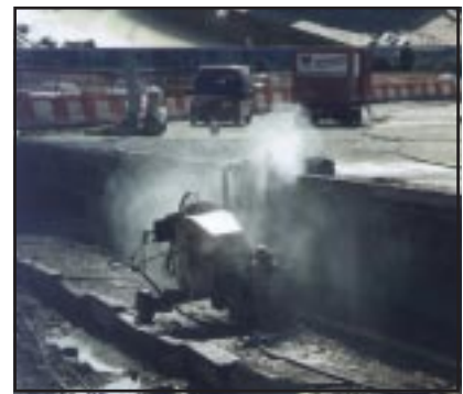
Robot 361 working supplied by the power pack.
