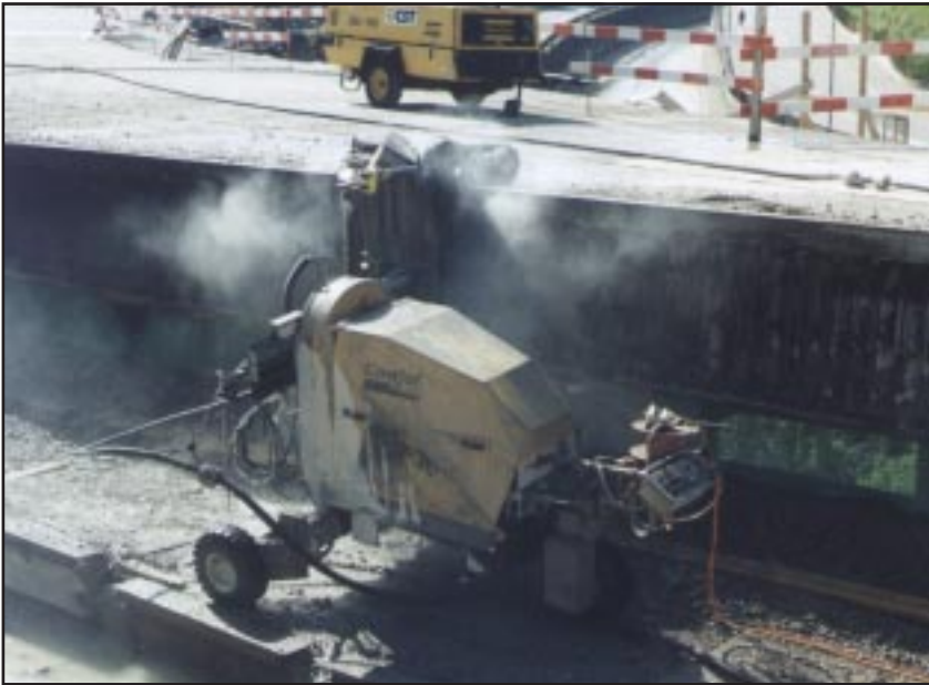
The Robot 361 working on vertical surfaces in the restoring of the Ponti Del Valico, Italy.
