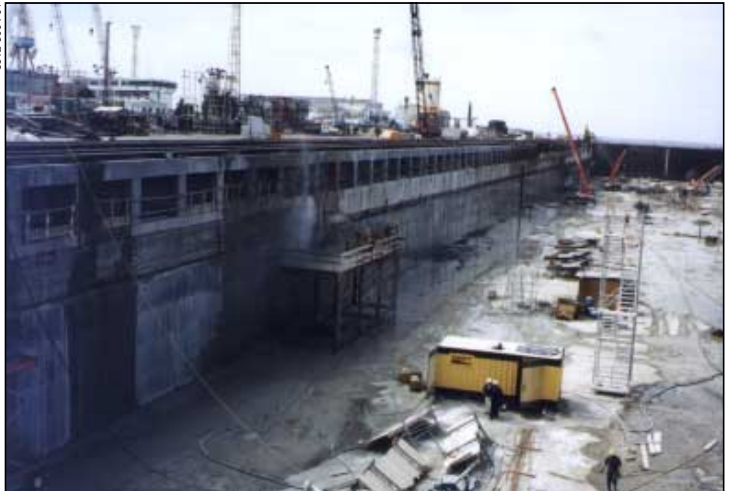
About 730m 3 of weak, porous concrete has to be removed from about 5600m 2 of the dock's high vertical walls.
