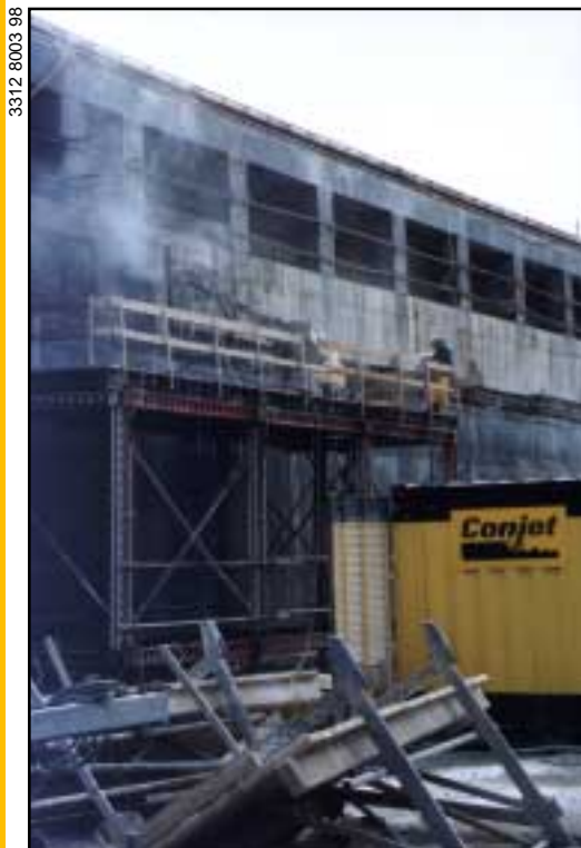
Contractor Belbetões is using its Conjet Robot 362 to selectively remove damaged concrete to a depth of 120mm to 140mm and below the
