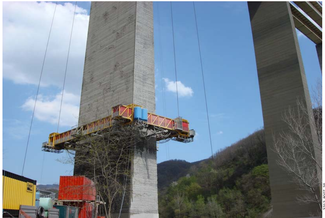
Repairs to the Rio Verde viaduct were performed from a special, purpose built cradle and working platform that wrapped round all four sides of the piers and supported by wire ropes connected to winches at ground level.
