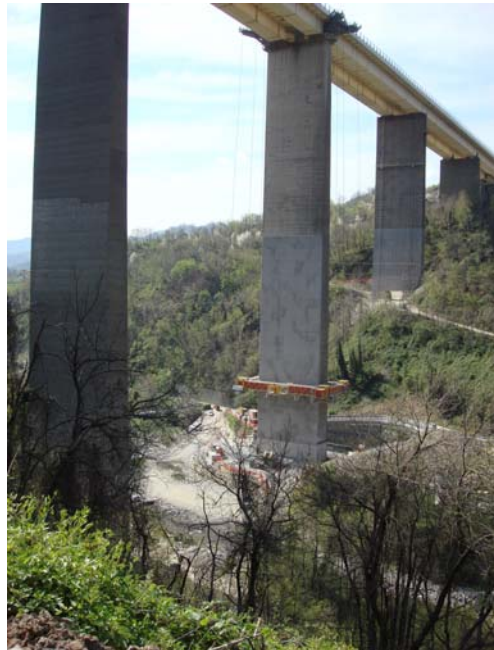
The Rio Verde viaduct is one of the tallest in Europe supported on piers up to 136m high and carries the dual two lane A15/E33 Autostrada della Cisa over a steep sided valley in the municipality of Pontremoli.
