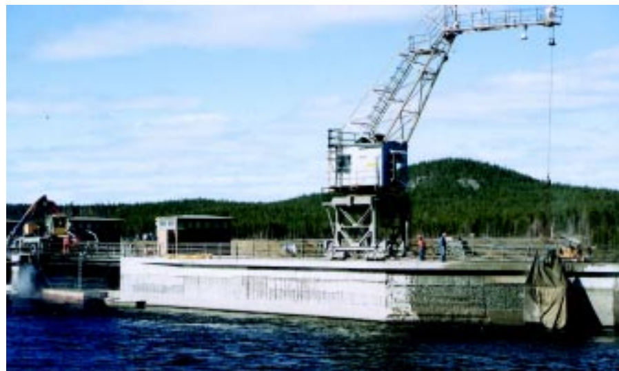
Conjet robot with vertical attachment operating from dam crest. Note debris catcher.
